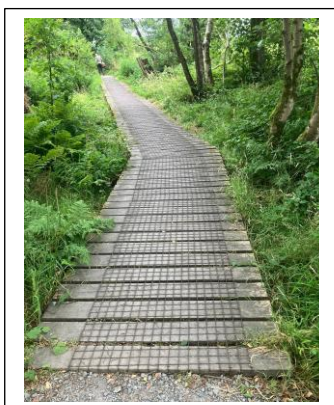
The existing boardwalk showing uneven boards
